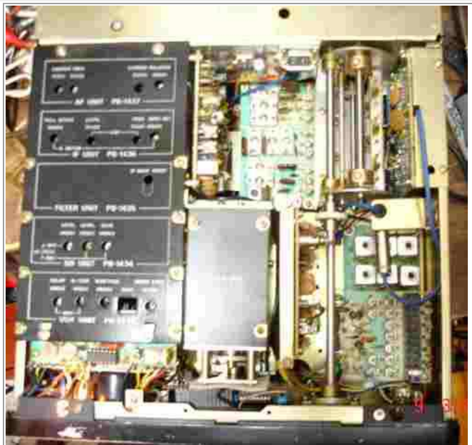
Top view of completed installation
